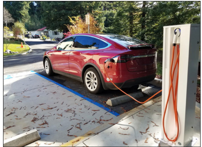
The new EV charging station at Humboldt State
