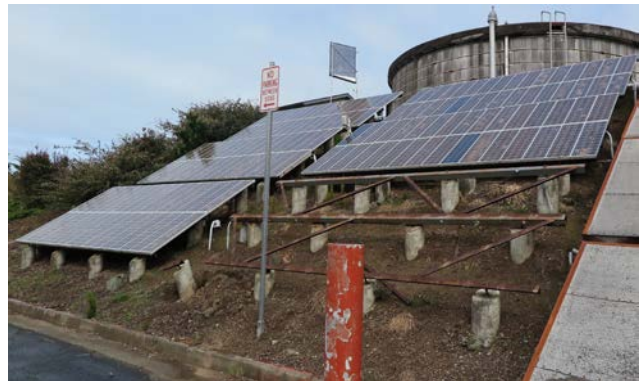
Fig. 1. A view of the array during decommissioning after two subarrays had already been removed (Photo Credit: Mark Rocheleau)
