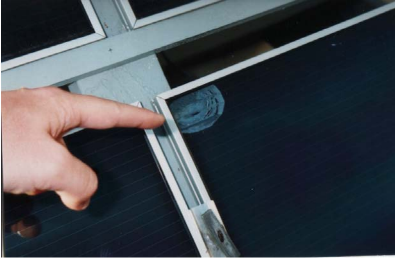
Figure 2. Water Intrusion Related Delamination in a Shenzhen Topray a-Si Solar Module.
