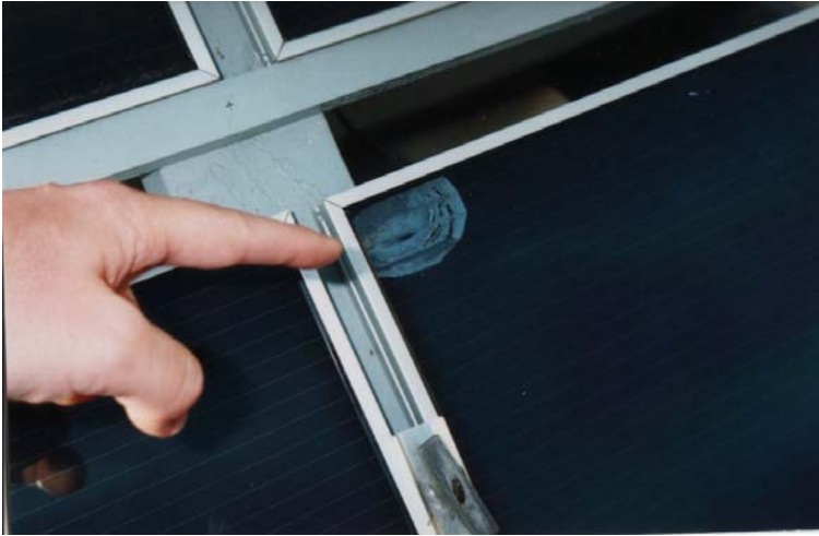
Figure 2. Water Intrusion Related Delamination in a Shenzhen Topray a-Si Solar Module.
